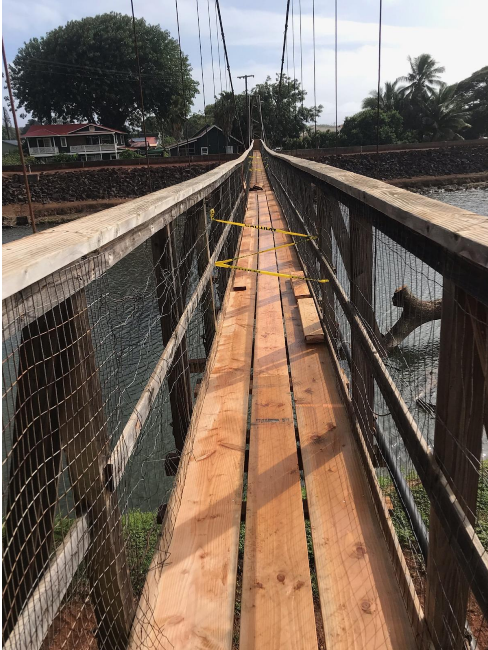
Photo caption: Runoff severely damaged the Hanapēpē Swinging Bridge on Christmas Day 2019.
