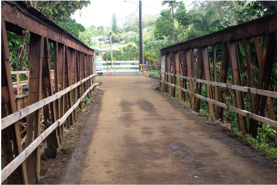
Photo caption: Closed since January 2020 for pre-construction work, the bridge is slated to open in September.
