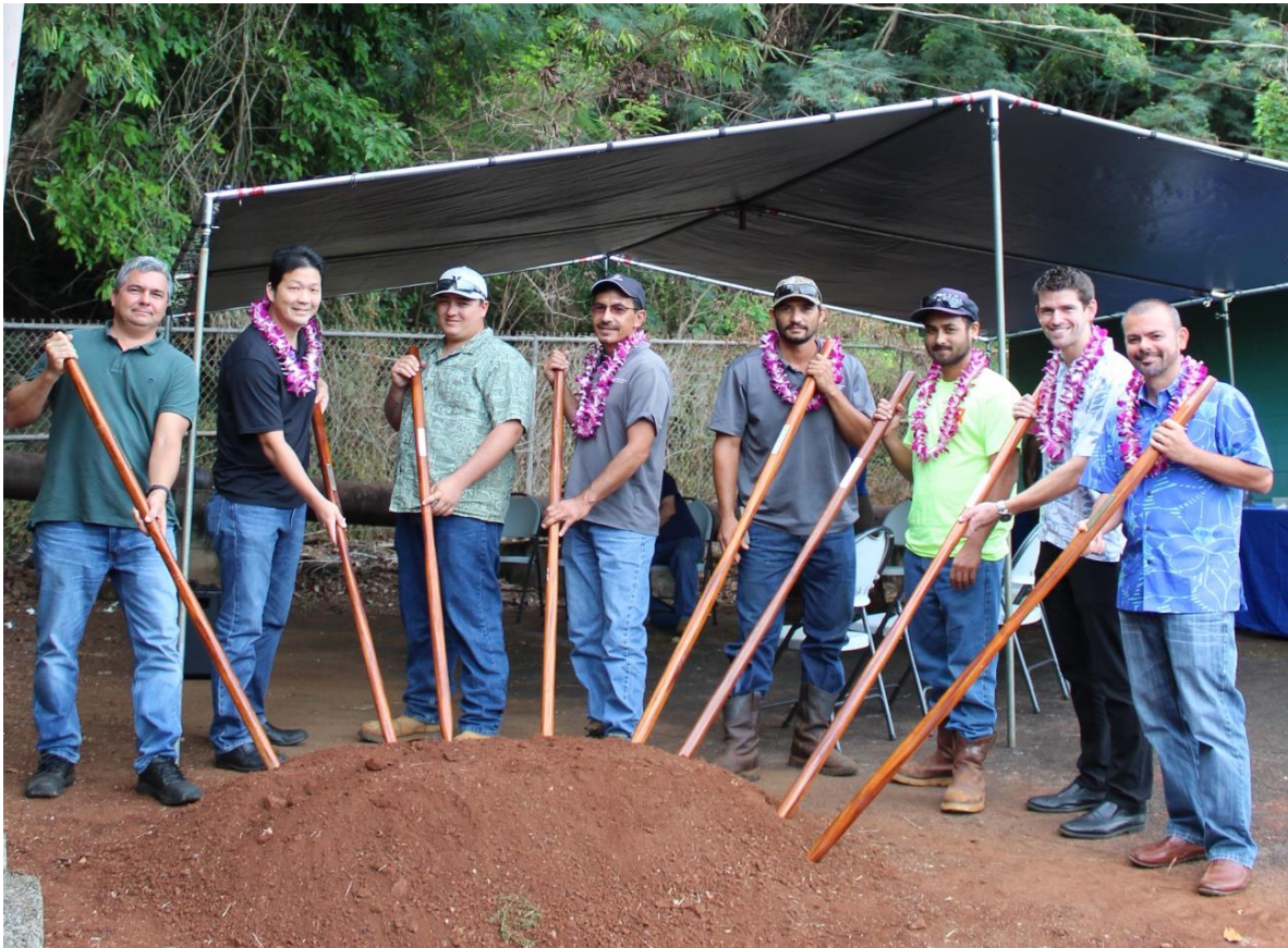
Photo by Department of Water: L to R: DOW's Claus Bollmann, Eric Fujikawa and Jet Levinthol, Wasa Electrical Services, Inc.'s Robin Perreira, Raym Jerves and Chad Manoi and the DOW's Bryan Wienand and Dustin Moises participate in the blessing ceremony for the Hanapēpē-Ele'ele Booster Pump Station Project on October 19, 2018.
