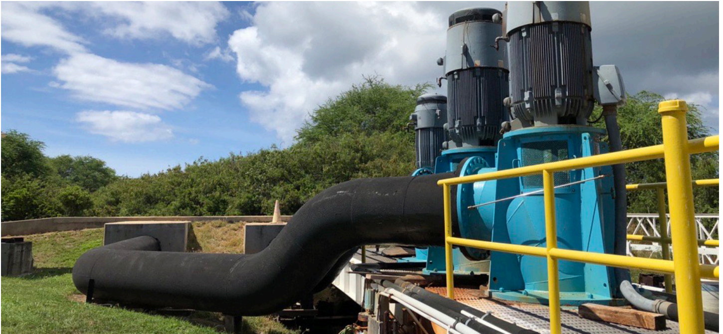
Water pumping station in Kekaha.
