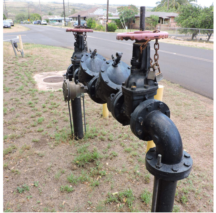
A water main in Waimea Town.
