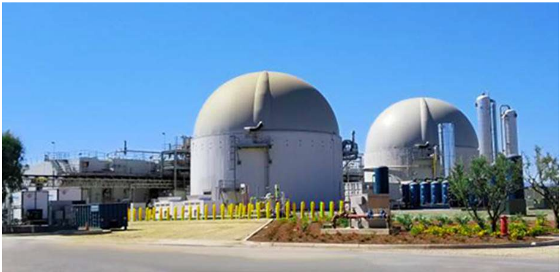
Figure 18: Vertical High Solids AD Plant, Perris, California
