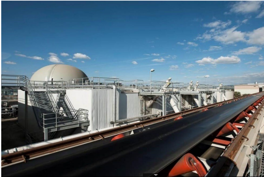
Figure 17: High Solids AD Plant, Perris, California
