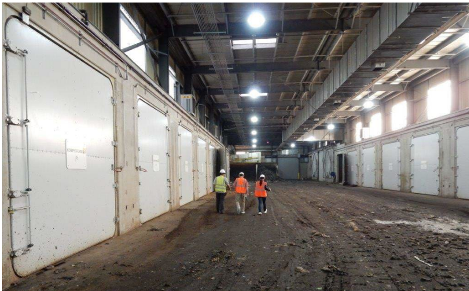
Figure 20: Interior of Zero Waste Energy Development Co. AD Plant, San Jose, California
