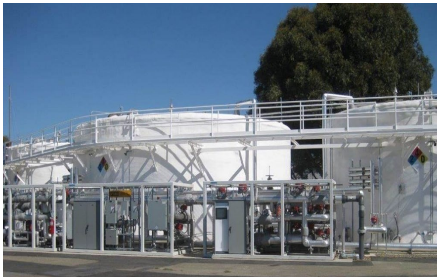
Figure 14: Low-Solids AD Plant, Sacramento, California
